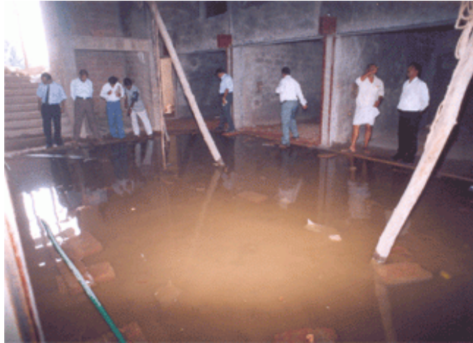
Water logging at construction site
